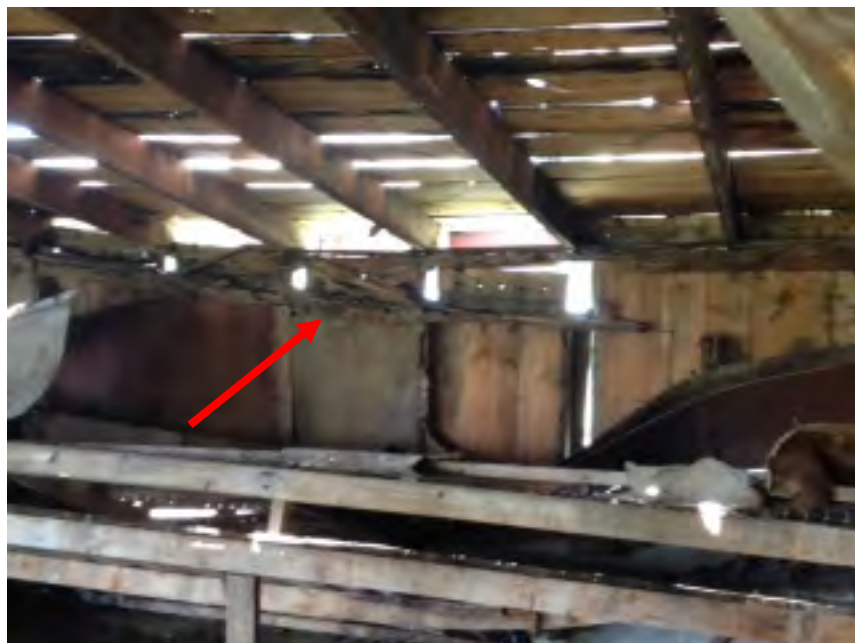
Figure 6 - Interior view showing the damaged structural supports and partially collapsed wall
