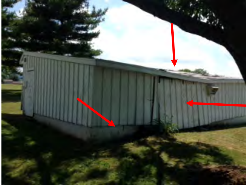
Figure 1 - Overview of the crumbling foundation, sagging roof, and collapsing wall
