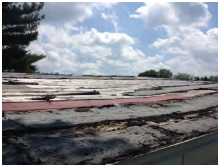
Figure 4 - View of the dilapidated roof
