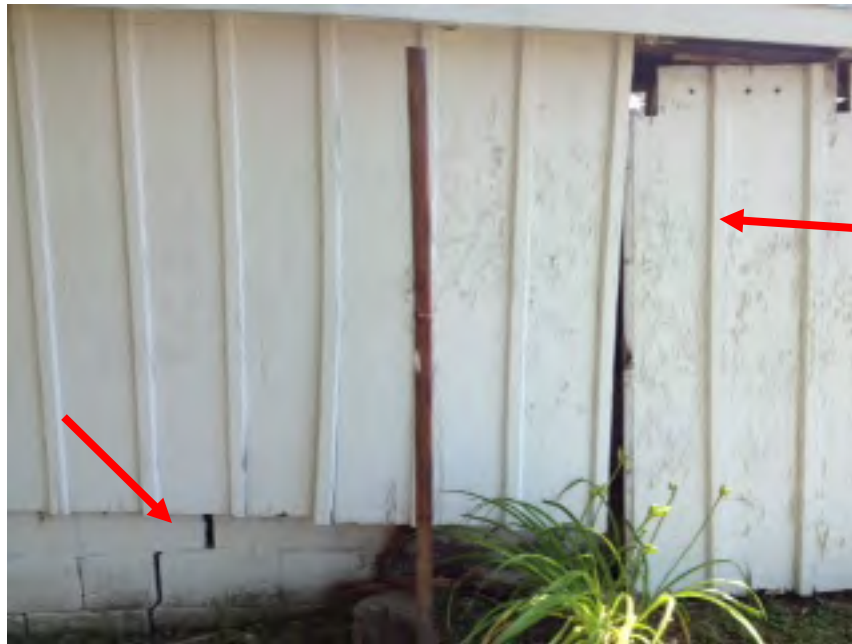
Figure 3 - Close-up view of the crumbling foundation and partially collapsed wall
