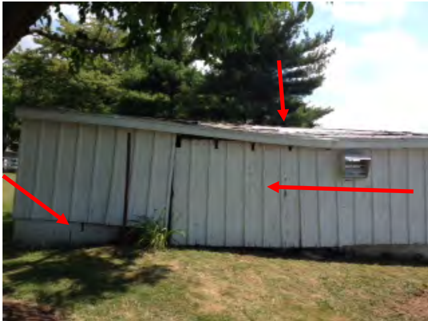
Figure 2 – Additional view of the crumbling foundation, sagging roof, and collapsing wall
