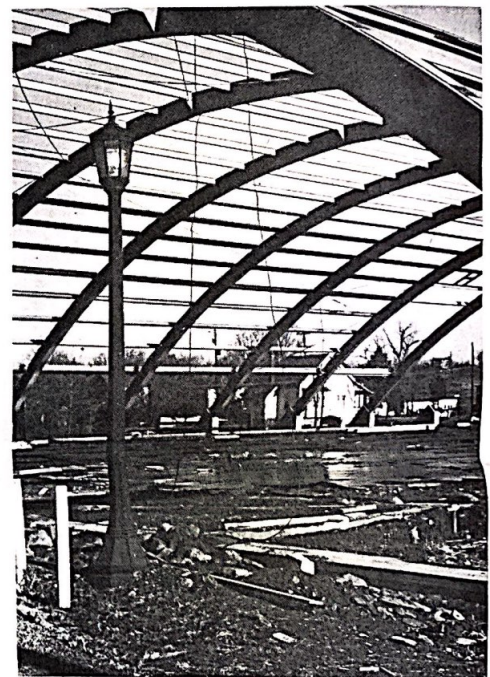
RAISED ARCHES of the new Koehler Field House confirm the construction that is being done on the upper part of campus.
