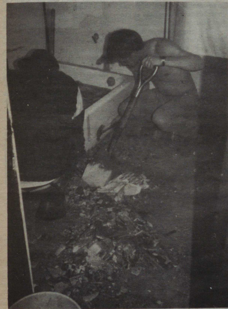
California University students repairing floor in a Chicago home during spring break. Photograph by the Rev. Cletus Hull.
