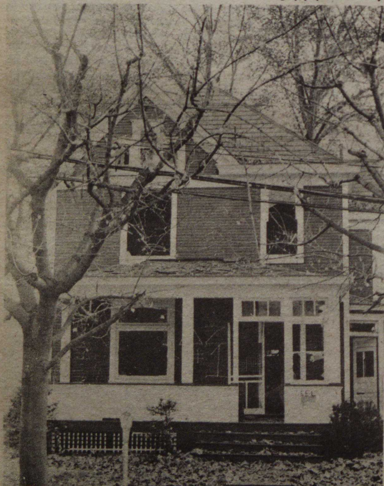
Now a windowless wreck, this house on Second Street was home for the Delta Zeta's for nineteen years.
