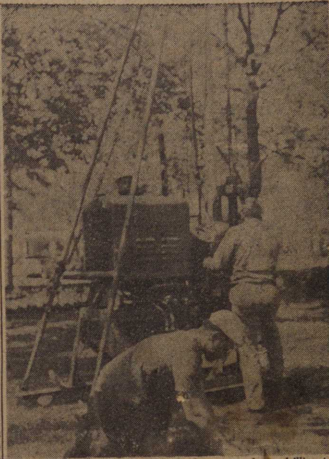
WORKING ON CSTC CAMPUS —Workmen are shown drilling to find secure foundation for new library building at California State Teachers College in front of Main Hall.
