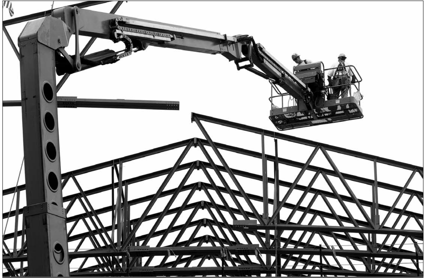
Two ironworkers bolt together the last truss at the top of the Convocation Center roof on Aug. 3, 2010. A pair of 300-ton cranes lifted a single 198-foot steel truss into place.
