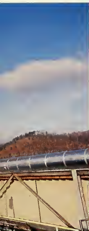
A fume incinerator destroys vent gasses from over 40 process vessels at Merck & Co., Danville.
