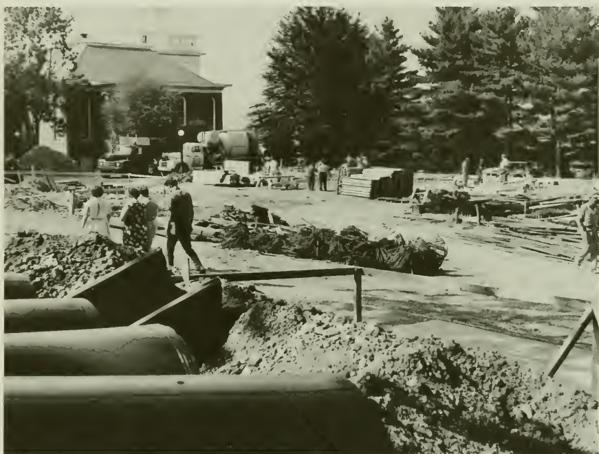
As Schuylkill Hall (West Hall) was being built between Carver Hall and Science Hall.
