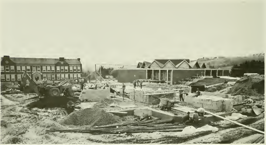
Construction of Bakeless Center for the Humanities, April 1969, with Navy Hall and Haas Center for the Arts in the background.
