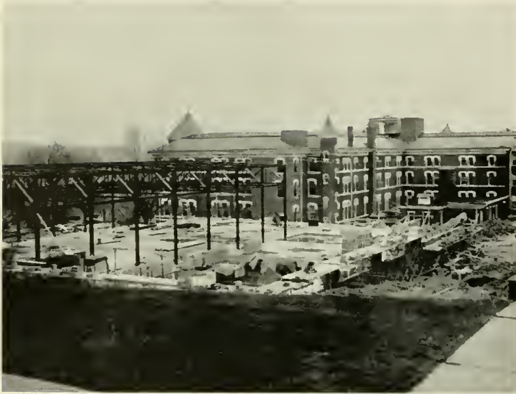
The rough stages of construction began to look like this in the spring of 1956.
