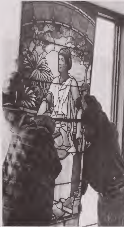
A NEW HOME FOR AN OLD TIFFANY Bud Smeenk (left) and Peter Koch (right) of Peter Koch Stained Glass in Williamsport install a panel of Tiffany stained glass window in the new library building. Koch's company has been contracted to clean and prepare the windows for installation in the new library.
