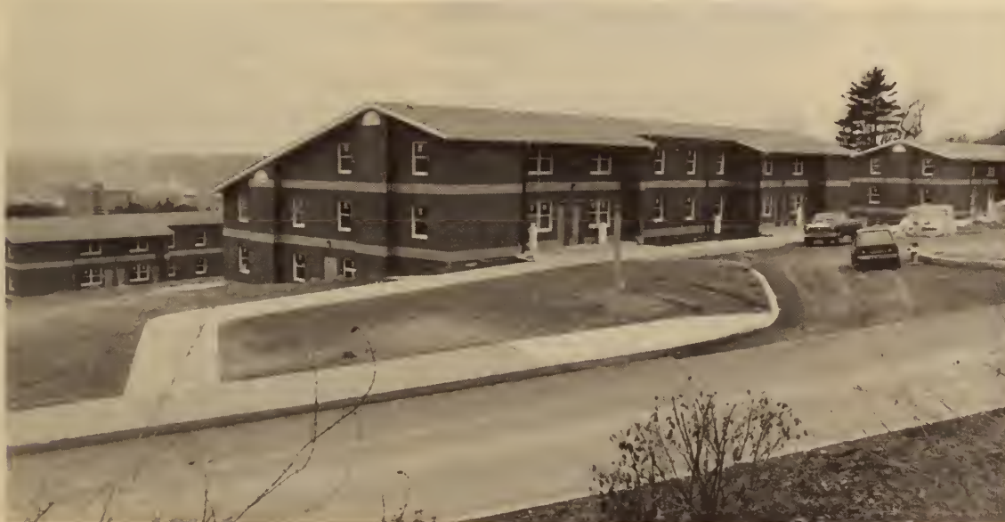
Construction continues on the housing units located on the upper campus. Each of the six buildings has 16 two-bedroom units. The student residence facilities will be ready for occupancy in the fall and will be open to 384 junior, senior, and graduate students.
