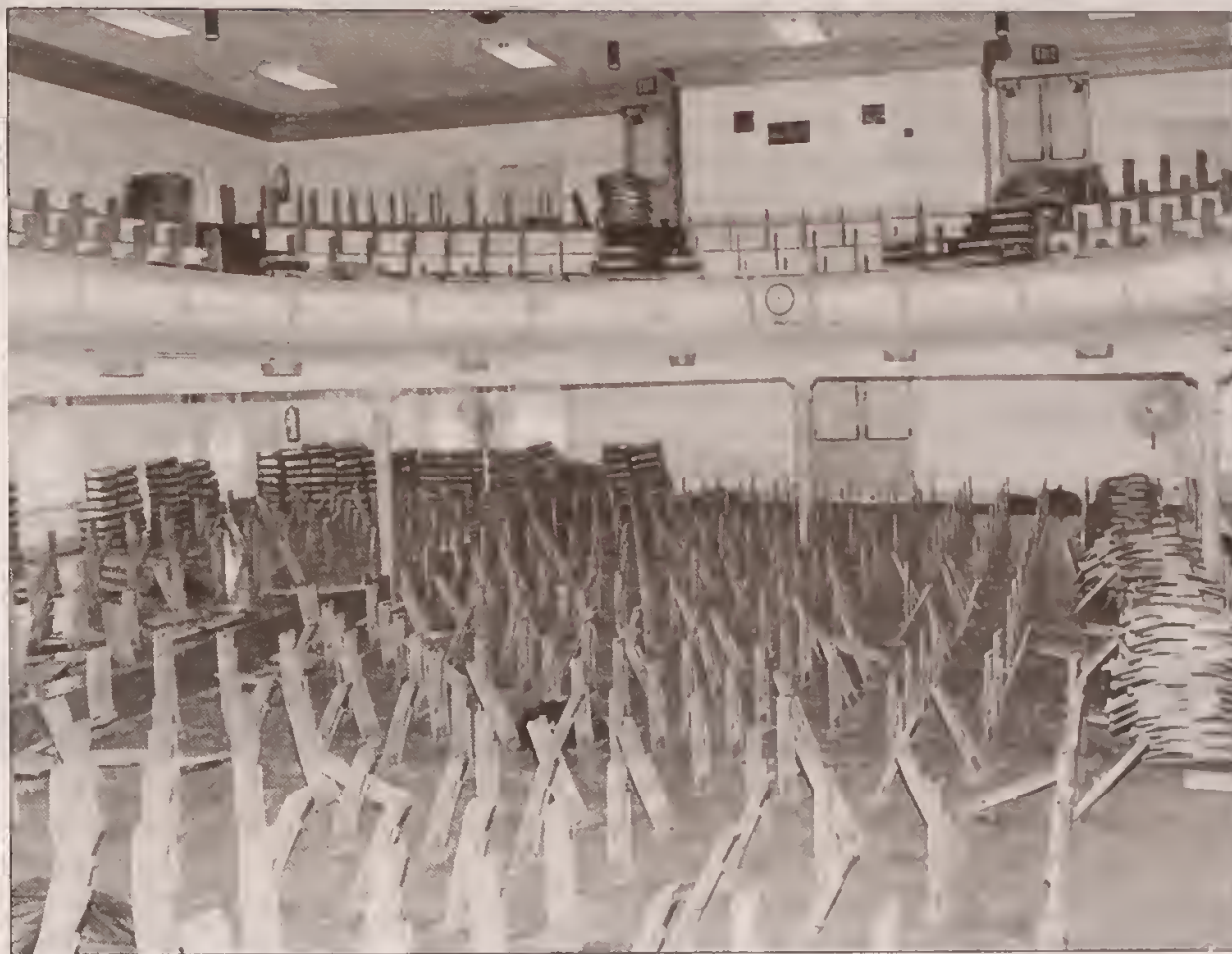
KENNETH S. GROSS AUDITORIUM, CARVER HALL: Major renovations are under way to replace the seating, carpeting, and house lights, upgrade the stage lighting, sound, and electrical systems, install air conditioning, and repaint the auditorium. A $100,000 gift last year from Kenneth S. Gross, together with additional funding through the Bloomsburg University Foundation, Inc., and Bloomsburg University have made this project possible. Completion is expected in 1993.
