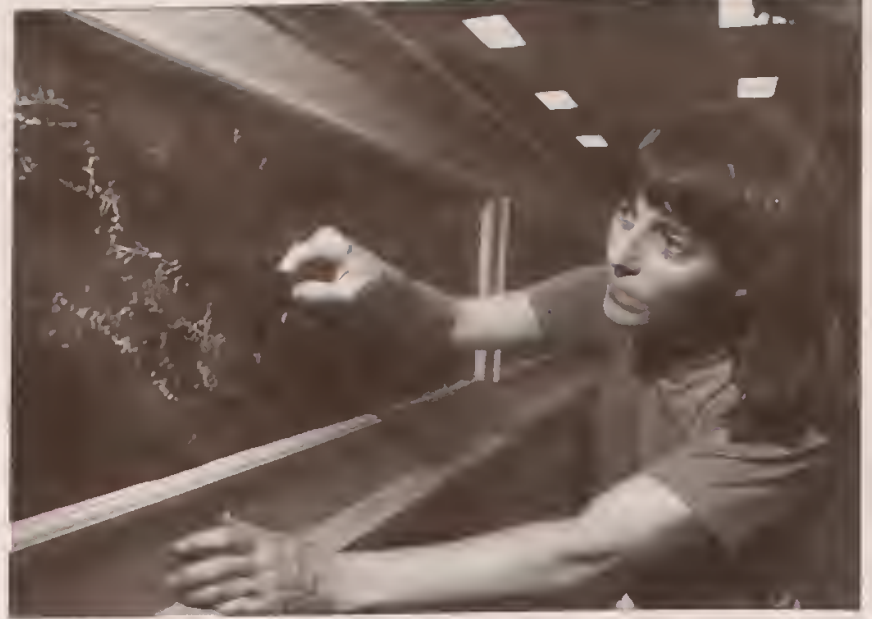
LIGHT TOUCH —Skilled artisan Marguerite Bierman uses a feather to create marbled surface on balcony panels at Kenneth Gross Auditorium, Carver Hall, as part of its restoration.
