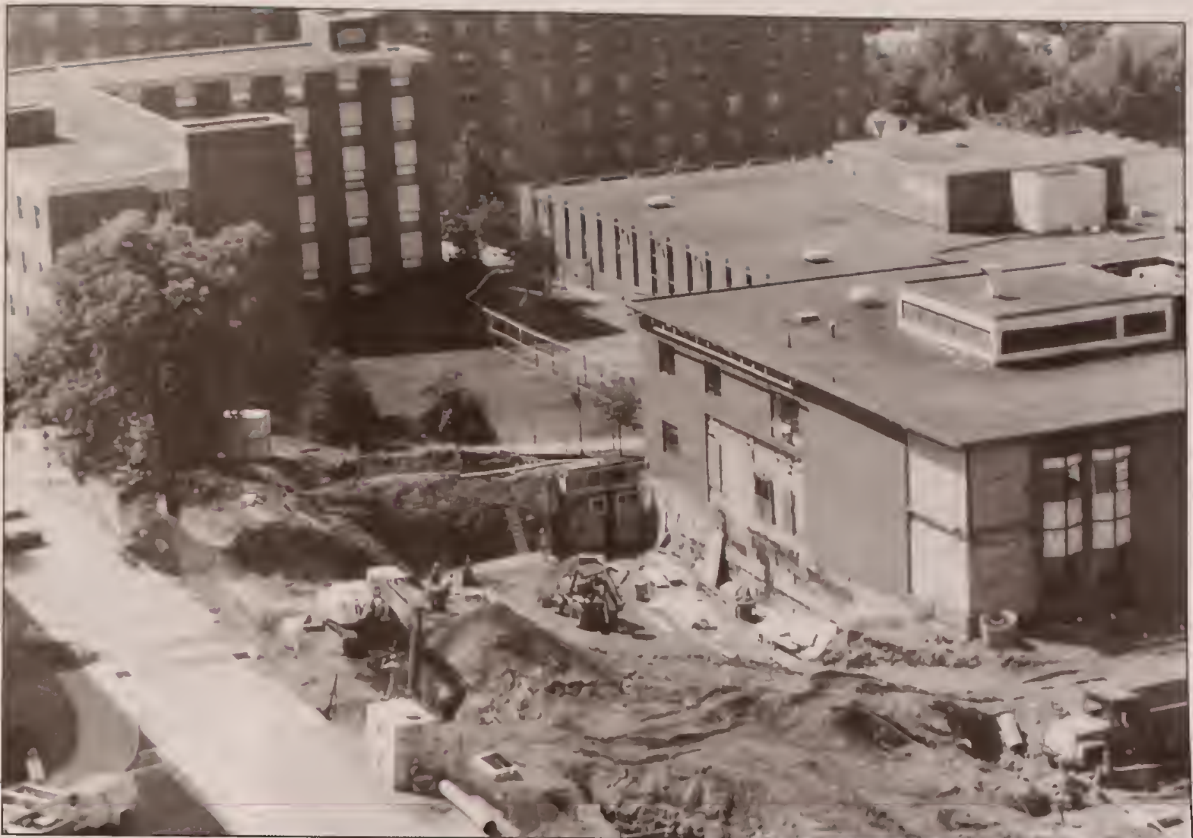
Work underway for addition to northeast corner of Kehr Union. In background: Lycoming Hall, Elwell Hall, and Scranton Commons.
