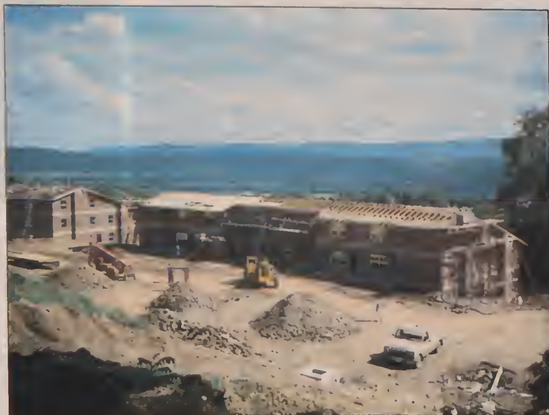
AHEAD OF SCHEDULE — Construction of a $5.35 million student housing project on the Upper Campus is ahead of schedule. The first of the six apartment buildings, containing a total of 96 two-bedroom apartments, may be finished in time for the spring semester. By the time the project is finished, it will provide housing for 380 students.
