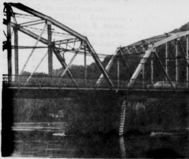
THE RIVER SUBSIDES - - Waters of the raging Susquehanna finally receded, but not before causing an estimated $5. million worth of damage to Clinton County. [Photo by DON D'INNOCENZO.]
