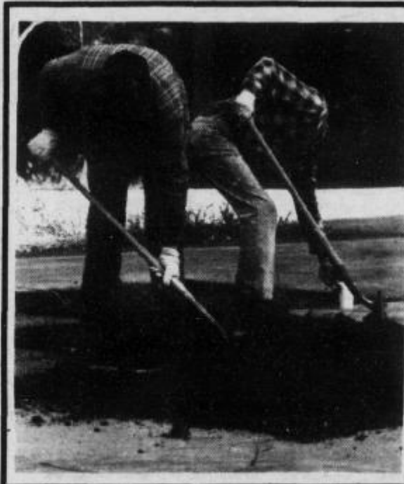
Workers dig up the soil outside of the Stevenson Library in preparation for the upcoming planting season.
