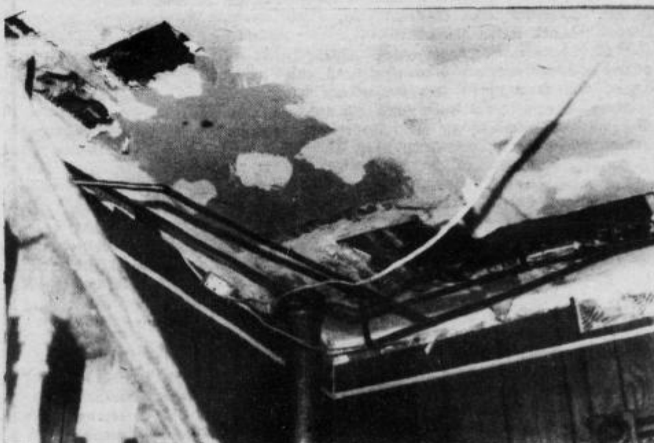
Pipes and wiring at the 424 West Water Street house that are exposed. The pipes and wiring hang down from the ceiling on the second floor.
