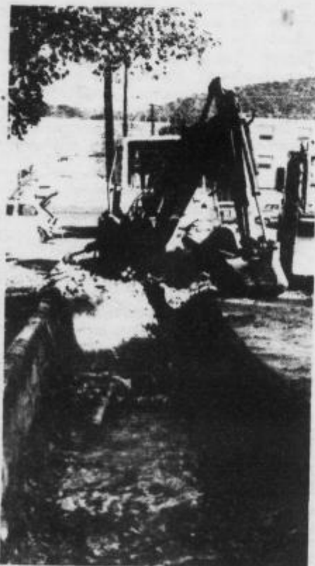
Workers tearing up Glen Road between Sullivan Hall and Bentley Hall to repair steamline.
