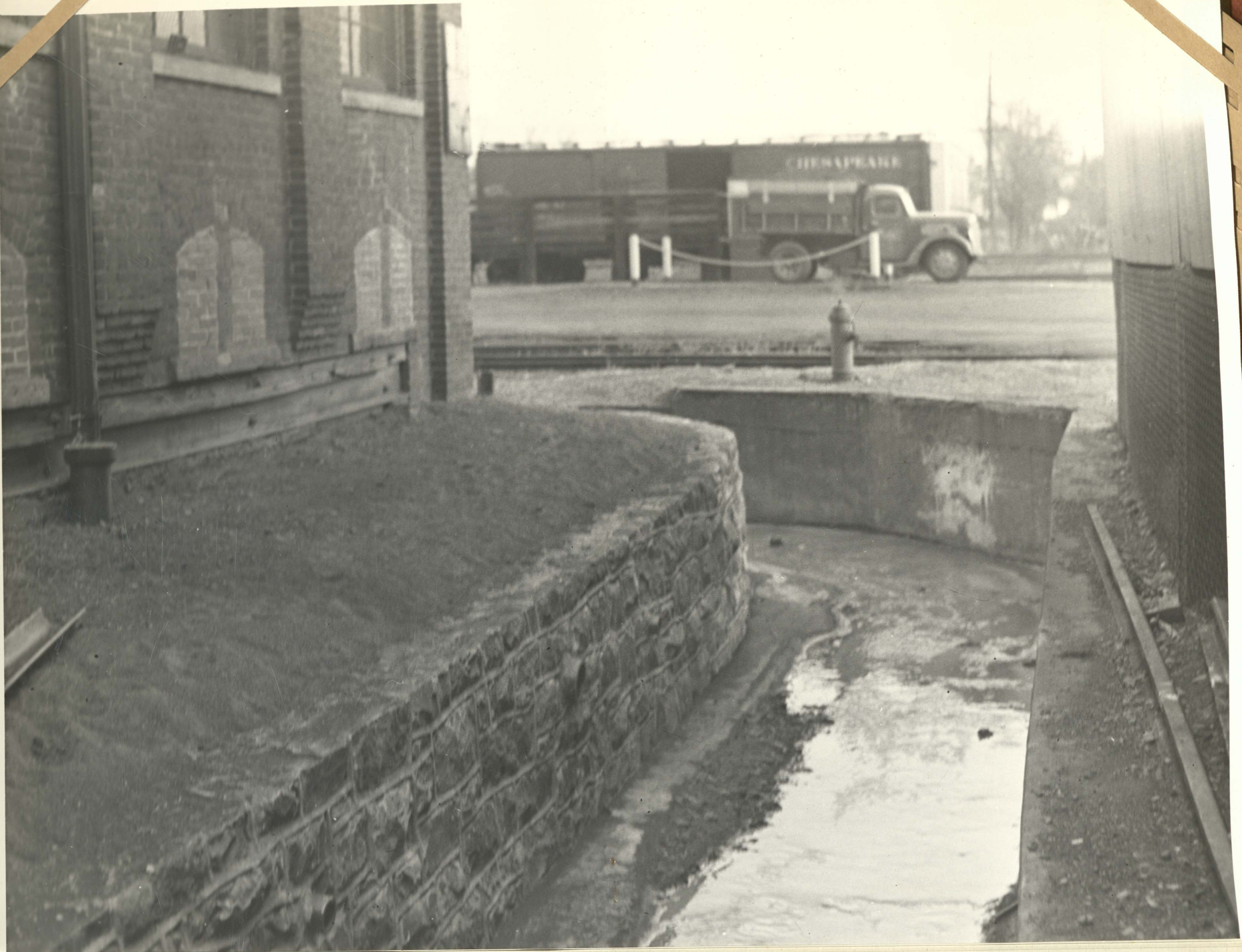
New stone wall erected in 1943 to protect the footing of building #5 from Snyder's Run.
